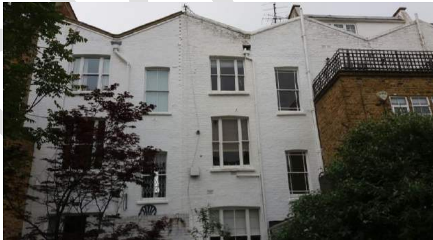
Prominent valley roofs, rear of Porten Road houses viewed from Ceylon Road.
