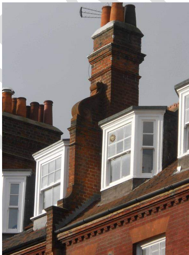
Distinct chimneys on nos. 53 to 59 and 40 to 62, Addison Gardens piers with scrolls.
