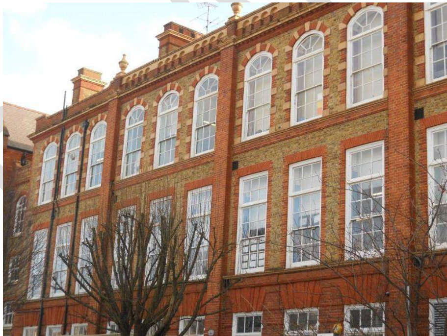
Elaborate cornice and parapet on Addison Gardens Primary School. Street trees along the perimeter enhance its setting.
