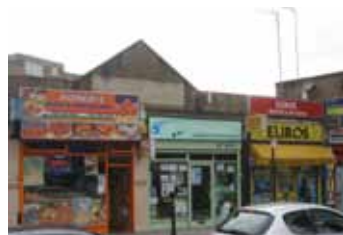
Figure 1.176: Poorly maintained shop fronts on North End Road
