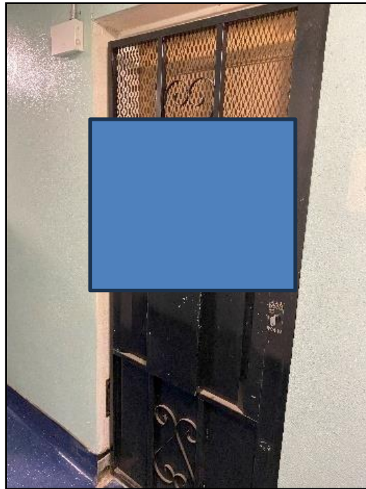
Security Grille And Old Flat Entrance Door (Flat xx) On Floor 8
