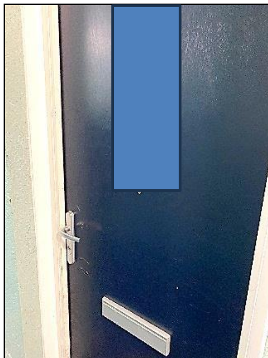
Damaged Flat Entrance Door (Flat xx) Below The Handle On Floor 5
