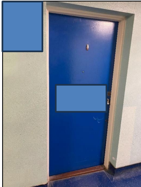
Damaged Flat Entrance Door (Flat xx) on Floor 4
