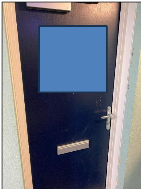
Damaged Flat Entrance Door (Flat xx) on Floor 7
